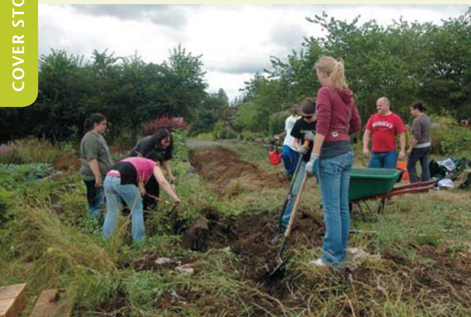
Young people work together for both hands-on teamwork experience and to change the directions of their lives. Here, kids are digging trenches for an automatic watering system.
